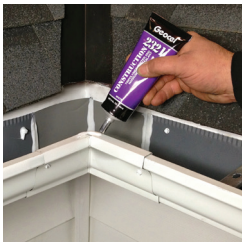
Apply a small amount of sealant to the top of the gutter on the front lip.
